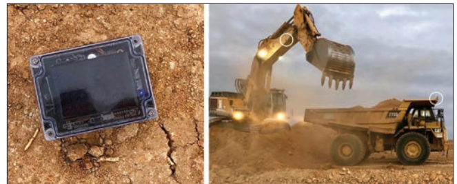
FIGURE 5. Left: picture of the smart node; right: smart nodes are mounted on the excavator and a truck; the locations are marked with white circles.
